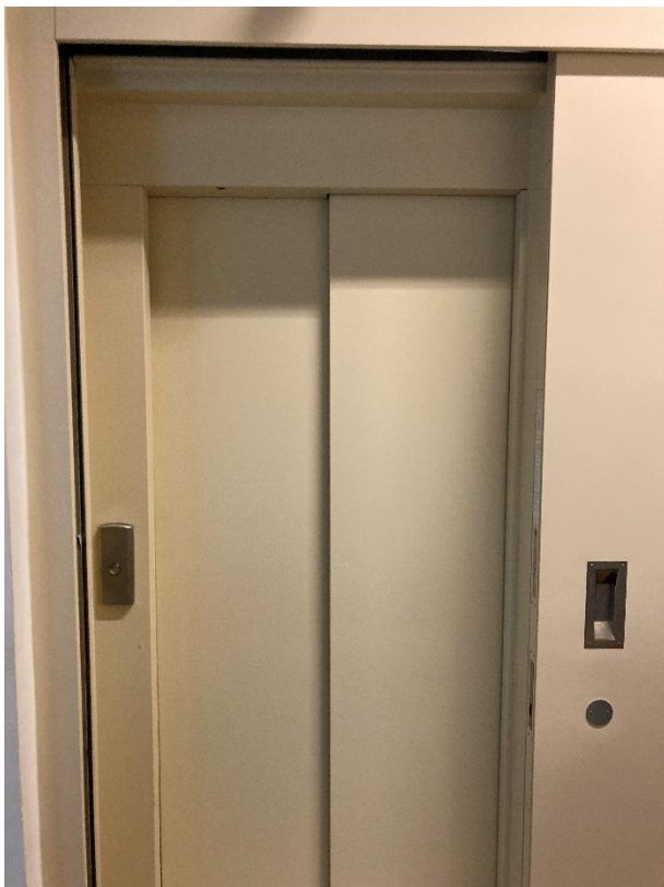
Figure 11: Lift doors on the mezzanine
