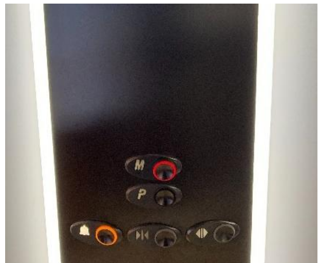
Figure 12: Control panel inside the lift on the mezzanine
