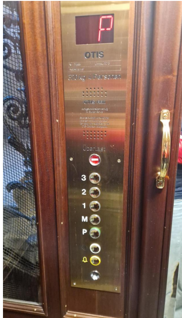
Figure 6: Control panel inside the lift
