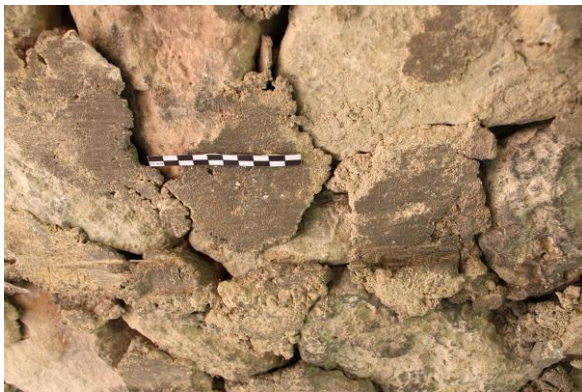
Fig. 20: black deposit / crust underside vault
