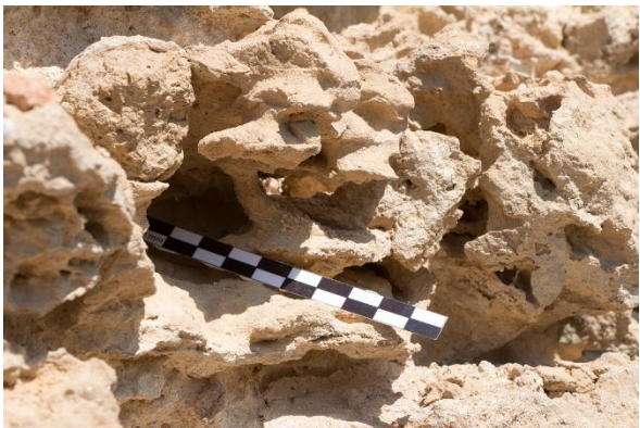
Fig. 16a: damages roman masonry, detail alveolisation masonry stone
