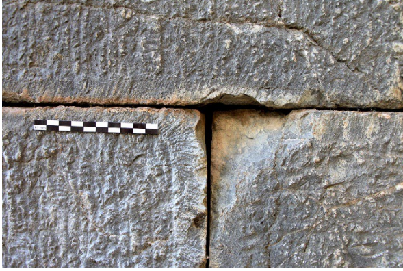
Fig. 31: Missing joint mortar, ashlar masonry, Water Temple
