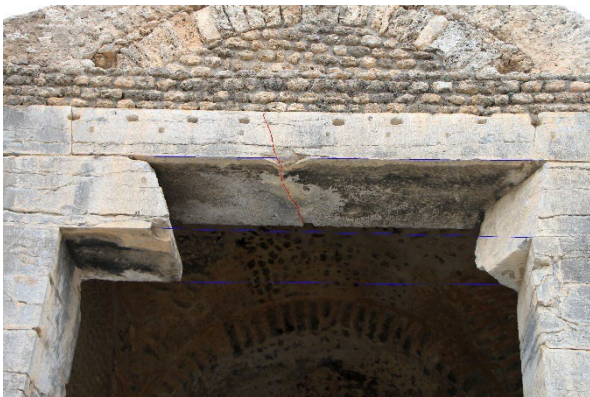
Fig. 27: Vertical crack, architrave / door lintel, Water Temple
