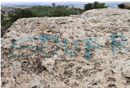
Fig. 29: Graffiti, roof cella exterior, Water Temple
