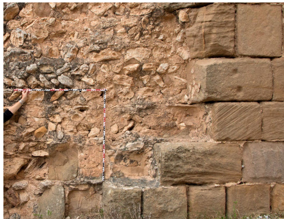
Fig. 42: Supporting walls, opus caementicium core faced with sand stone ashlar blocks, Aqueduct
