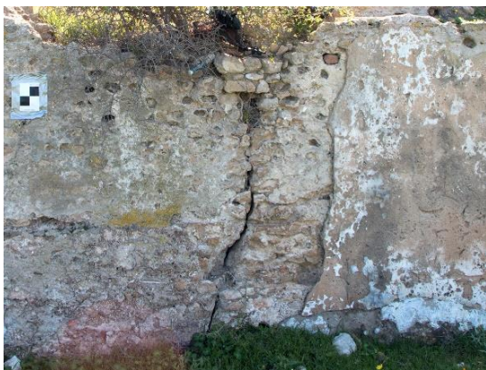
Fig. 22: vertical crack north side
