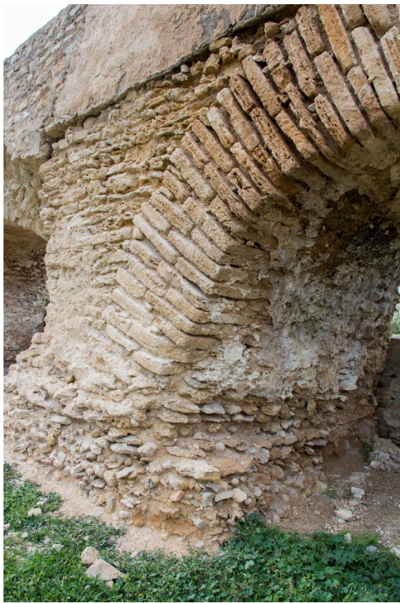
Fig. 4: aqueduct, preserved antique vault between pillar P8-P9 in the foreground and robbed vault in the background
