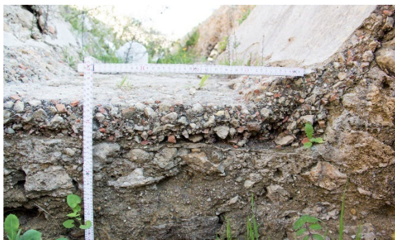
Fig. 6: cistern, drain channel between compartments between 8 and 9, structure and thickness of different plaster layers
